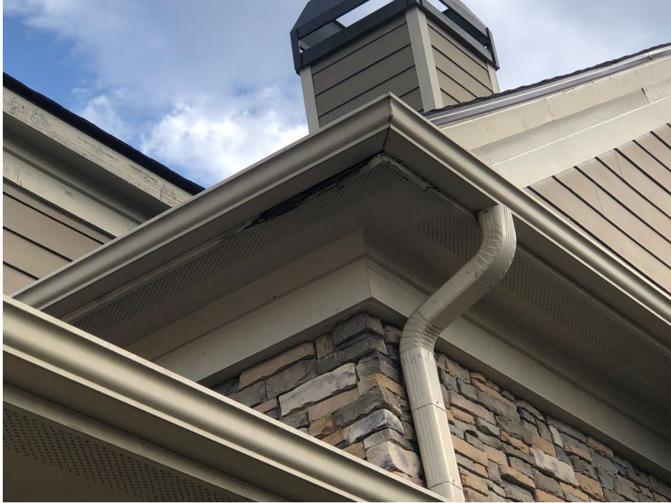
27. View of a typical damage soffit at the clubhouse.
