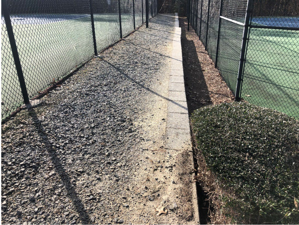
11. View of silt accumulation above the retaining wall displacing the blocks.
