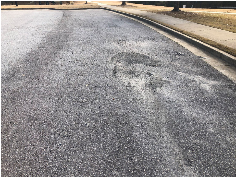
2. View of settlement and loose aggregates at the private parking lot.
