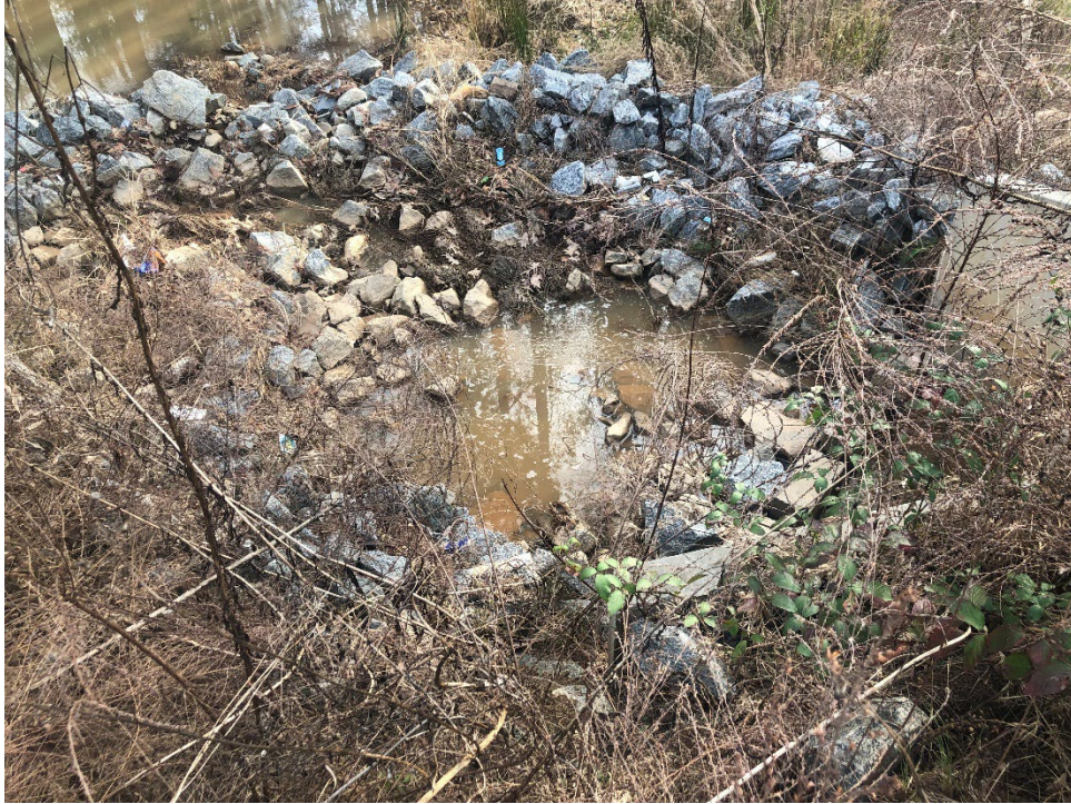
15. View of displaced rip rap and water ponding at the outlet culvert of the detention pond.
