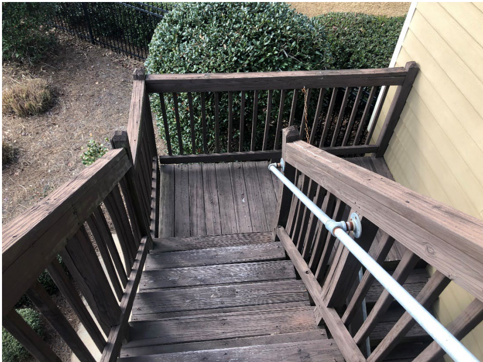
34. View of the stair that is structurally compromised.
