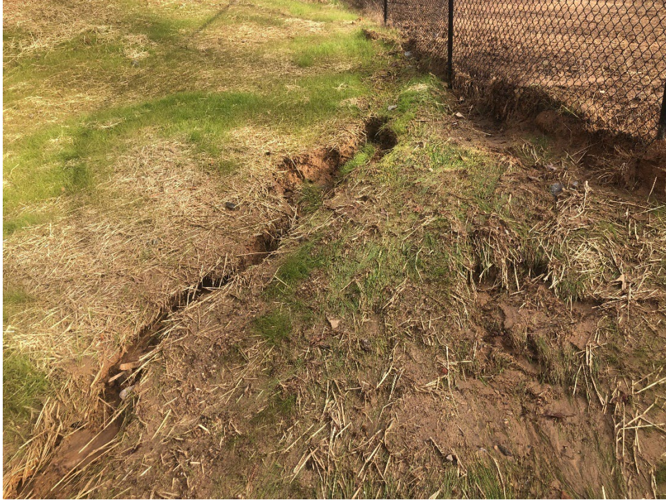
17. View of rill erosion at the detention pond.
