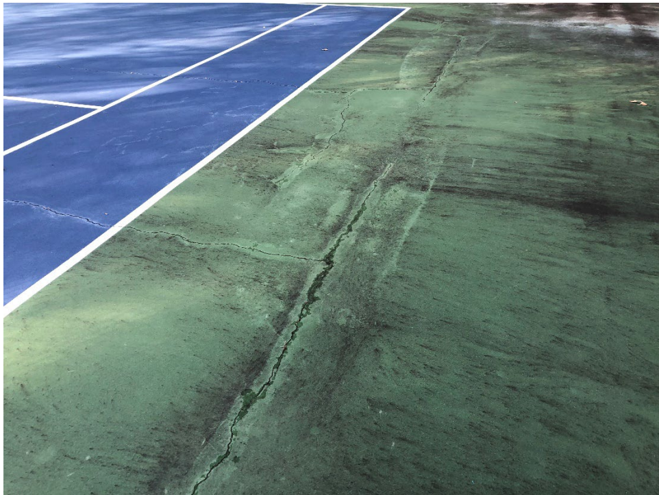
24. View of a typical crack at the tennis court.
