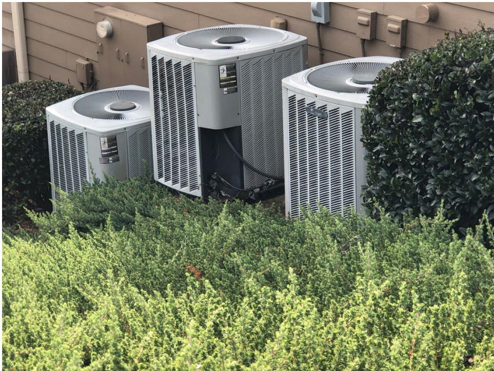
36. View of the typical HVAC units.
