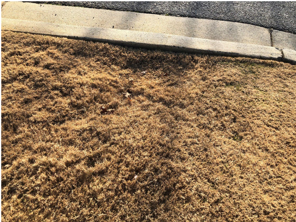
12. View of a sinkhole behind the concrete curb at the entrance of the clubhouse.
