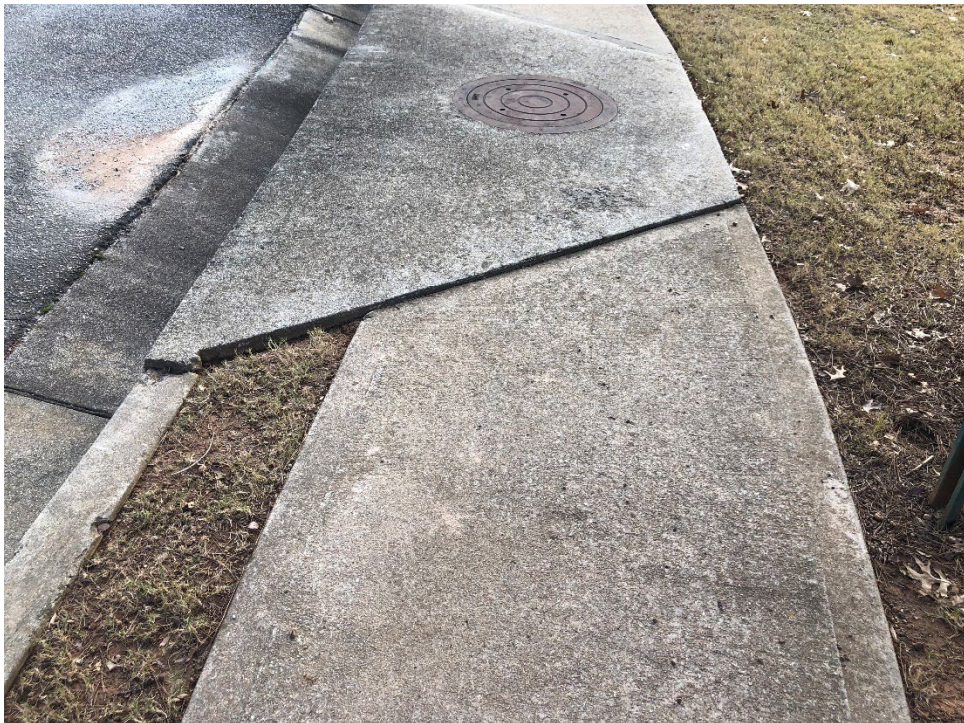
6. View of a settled sidewalk.
