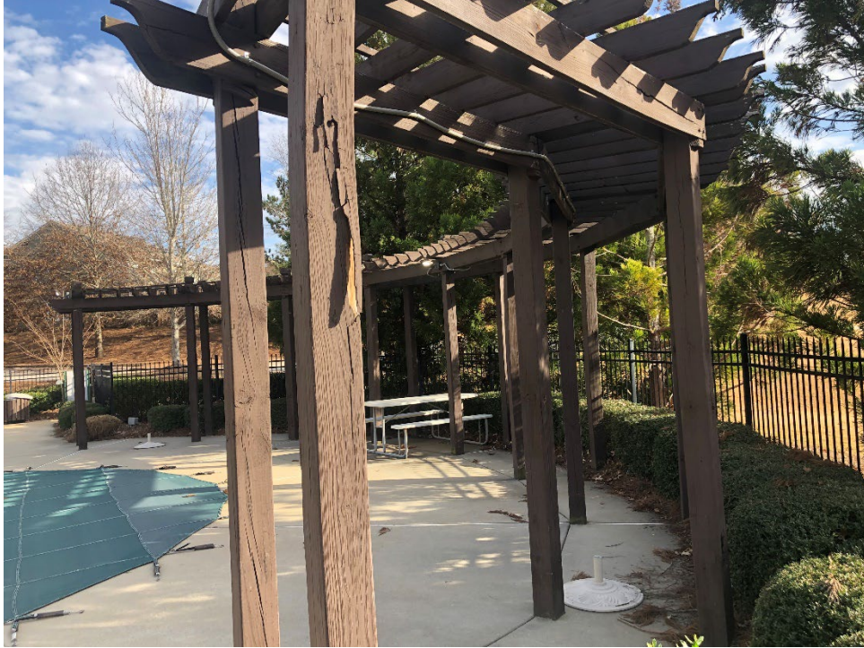
35. View of a damaged column and fading paint at the arbor.
