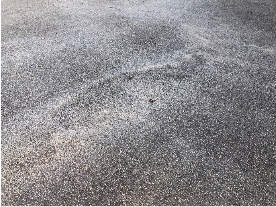
1. View of loose aggregates at the private parking lot.
