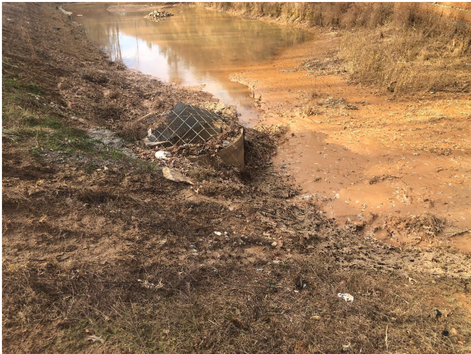
14. View of water ponding and heavy silt accumulation at the detention pond.
