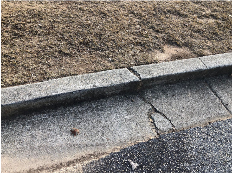
4. View of a typical crack with cracks and spalling concrete observed.
