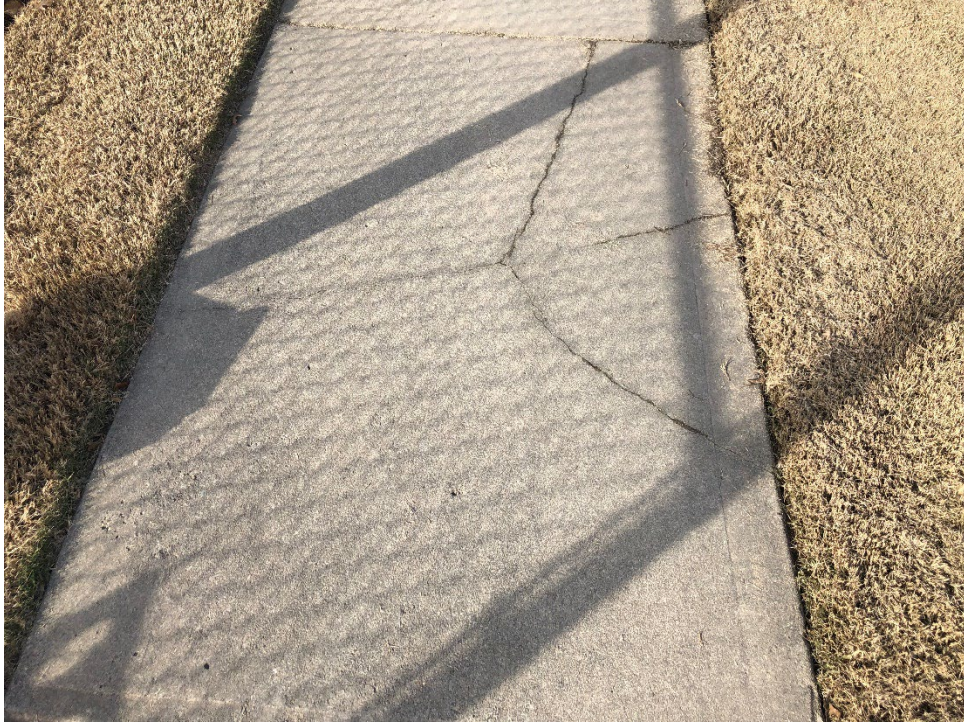
5. View of typical crack at the sidewalks.
