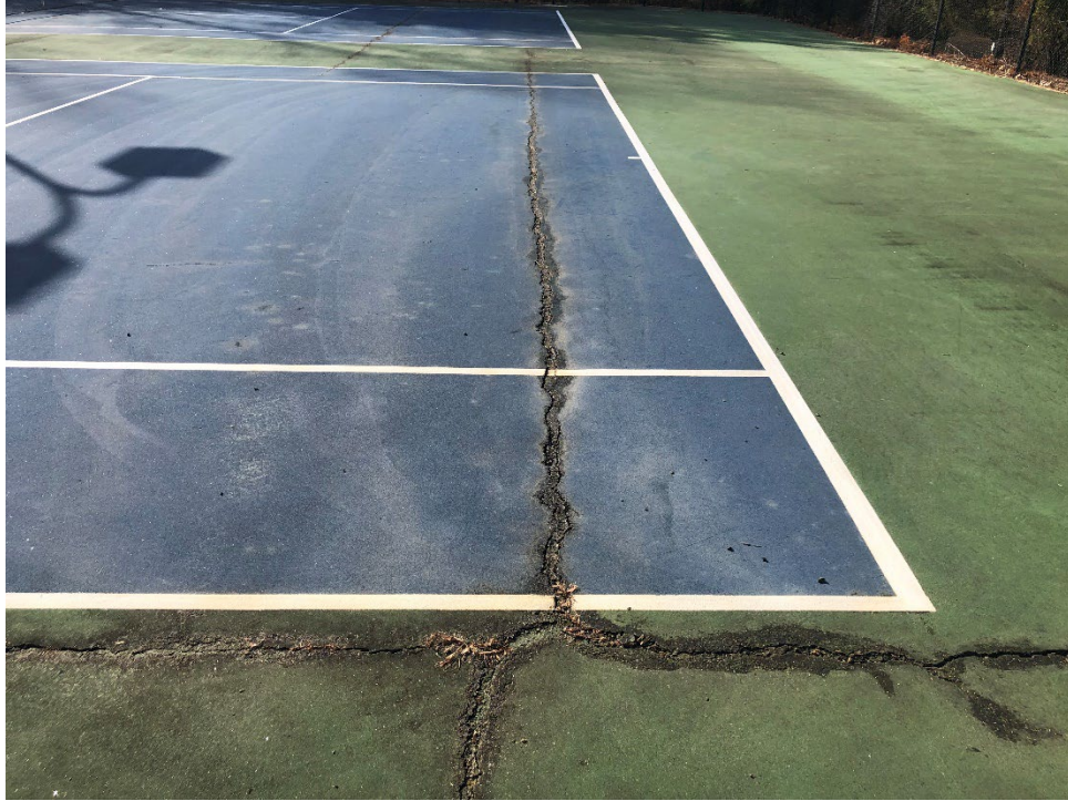
25. View of typical cracks at the tennis court.
