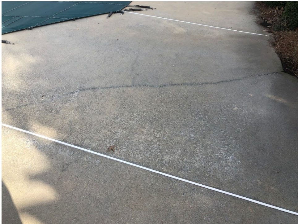
22. View of a crack at the swimming pool deck.
