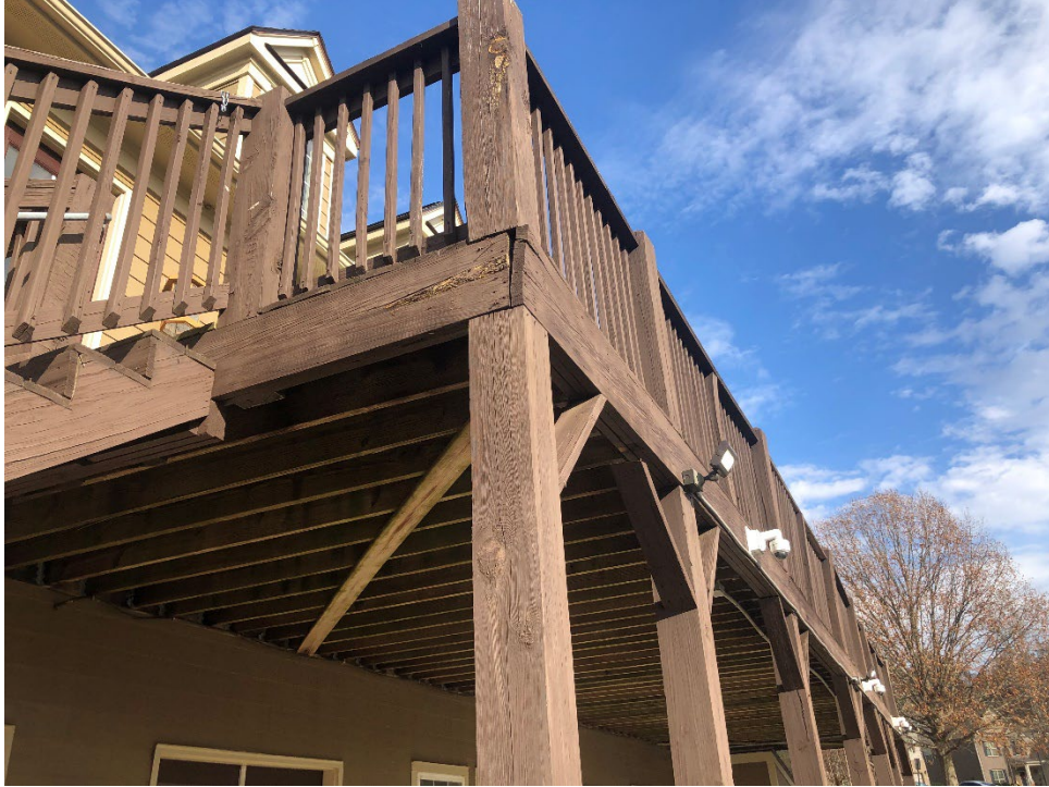
33. View of the deck that is structurally compromised.
