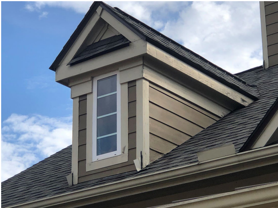
28. View of a typical damaged trim and fascia at the clubhouse.
