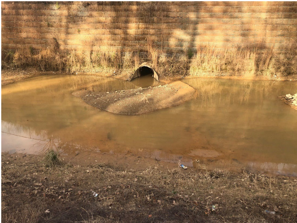
16. View of heavy silt accumulation and lack of rip rap at the detention pond.
