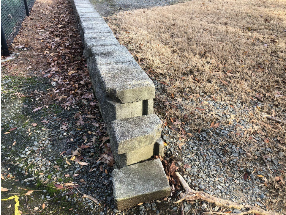
9. View of loose and displaced modular blocks at the retaining wall.
