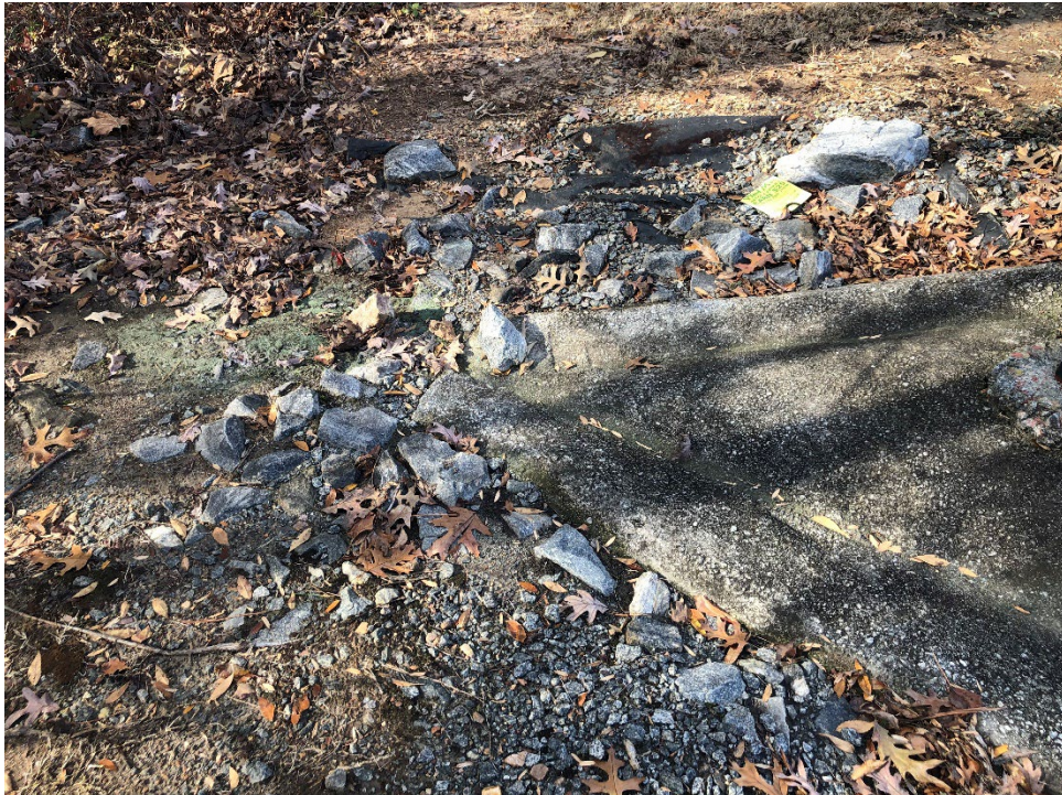
10. View of exposed filter fabric, displaced river rock and exposed soil.
