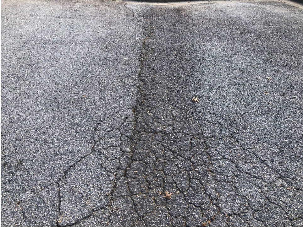
3. View of a typical "alligator" cracked at the private parking lot.
